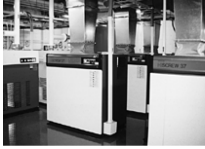
Fig. 4 Outside view of air compressor system
