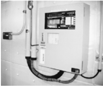
Fig. 5 Control board for controlling the number of compressors
