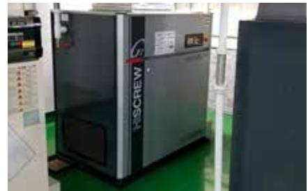
Compressors at the Fujiyama Works
