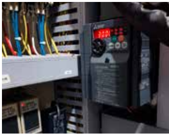
Optimal control of pumps using inverters
