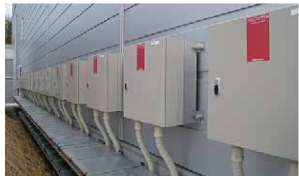
PV Inverters at Fujiyama Works
