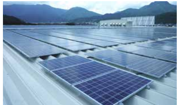
Solar panels at Logistics Center
