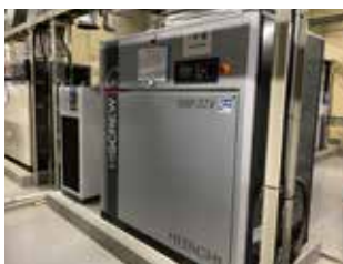
Compressors at the Kangawa Works
