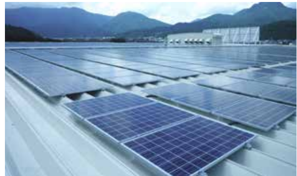
Solar panels at Logistics Center
