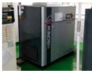
Compressors at the Fujiyama Works
