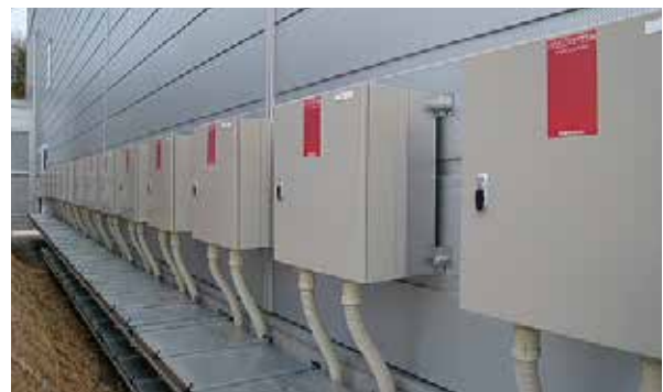
PV Inverters at Fujiyama Works
