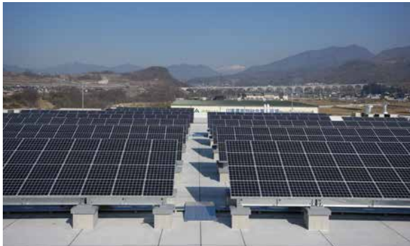
Solar panels at Kangawa Works
