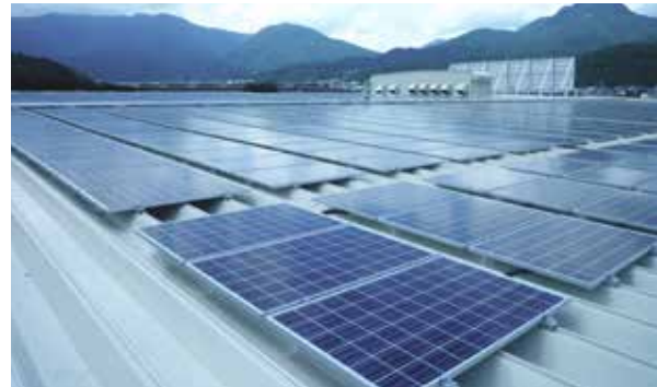
Solar panels at Logistics Center
