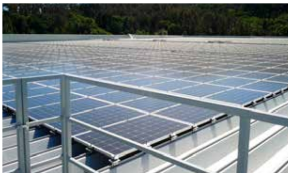
Solar panels at Fujiyama Works
