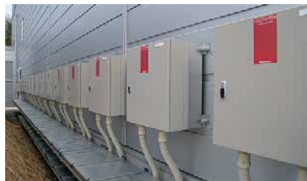
PV Inverters at Fujiyama Works
